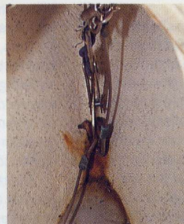
This makeshift lower forestay attachment can cause misalignment and excessive wear
